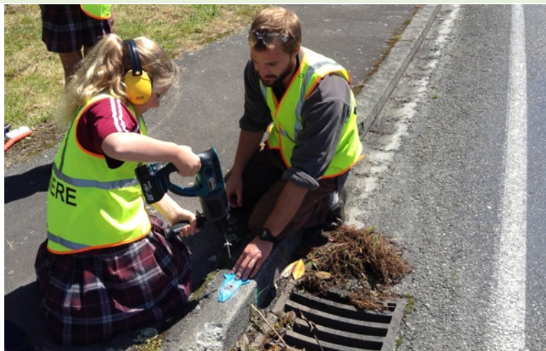
Above: Charlotte Sweeney & Lyndon Slater (DOC) installing a plastic fish in Kanieri
